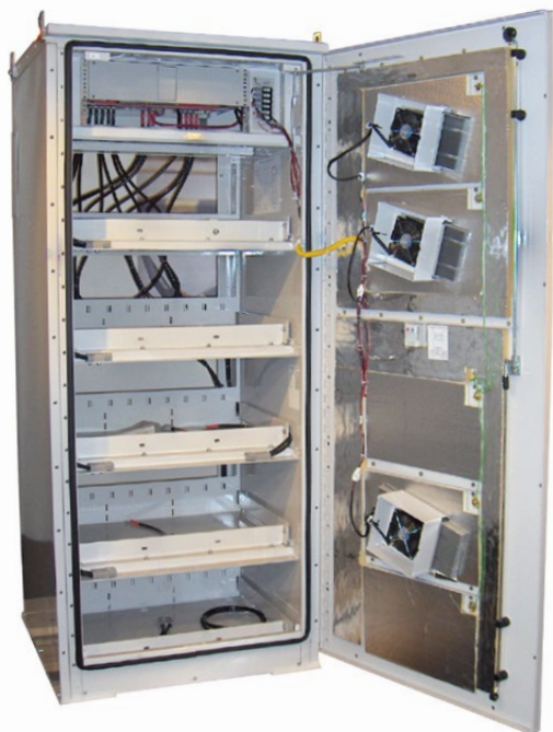
10.15: Integrated cell site battery-only cabinet
