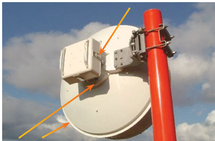
8.18: Example of RF leakage in a noncompliant microwave antenna
