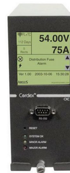
10.11: A system controller interface displaying voltage, amperage and alerts
