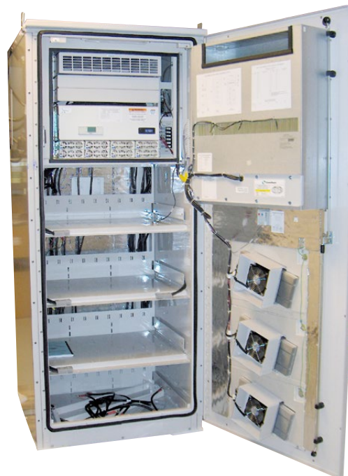
10.16: Integrated cell site power and battery cabinet
